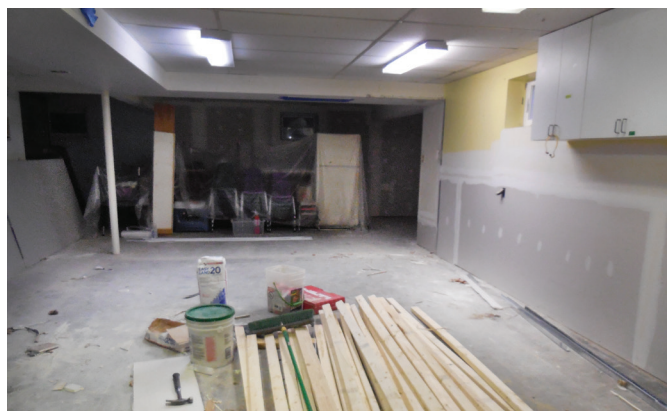
A view of the gutted classroom mid-repair, due to devastating county sewage back-up.
